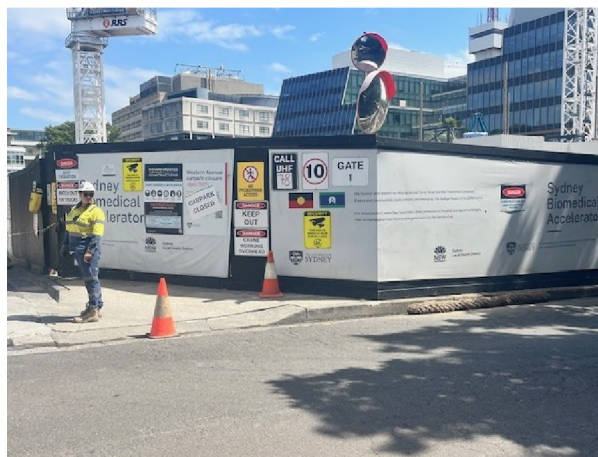
Photo 15: Compliant notice displayed at the main site entrance; No signs of tracking onto surrounding roads
