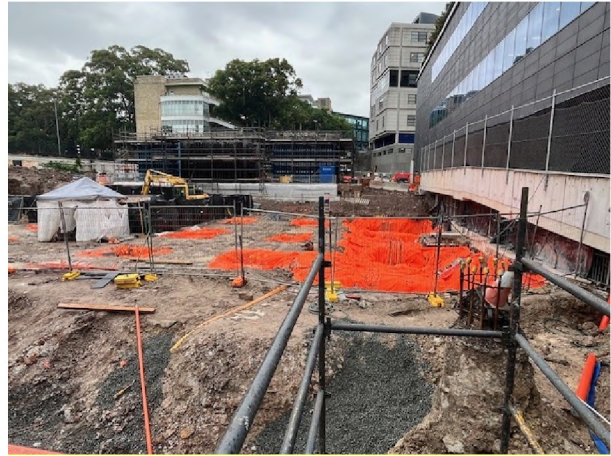
Photo 12: The asbestos containment zone remained in place with asbestos fibre air monitoring ongoing
