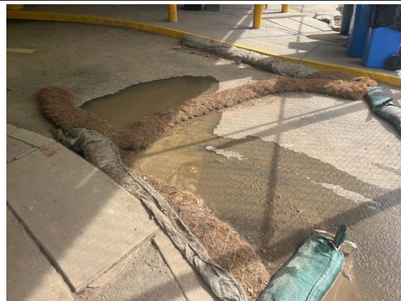
Photo 24: A gurney was in use at the heavy vehicle access, risking discharge of sediment-laden water to stormwater
