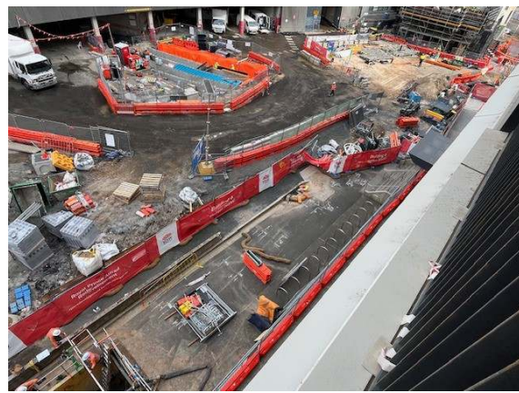
Photo 14: Royal Prince Alfred Hospital (H1) to the west of the site, and stormwater works (under the REF)
