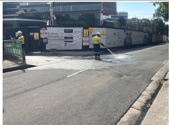
Photo 25: A hose was also in use at the site entrance, risking discharge of sediment-laden water to stormwater
