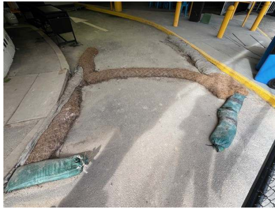
Photo 22 & 23: Coir logs and ERSED controls around the stormwater drain at the site compound / carpark entrance required replacement
