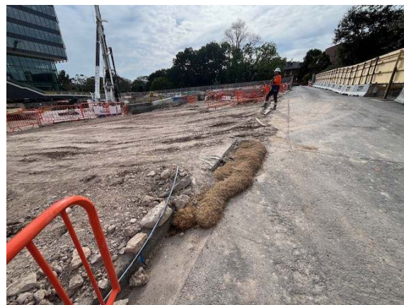
Photo 18: Heavy vehicle access to the main site – no wheel wash in place and tracking evident
