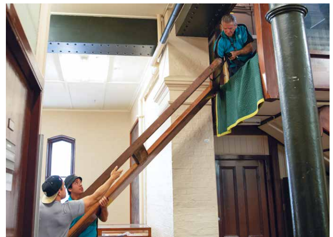
Gynea Removals carefully move the cabinet sections through a hole made in the staircase
