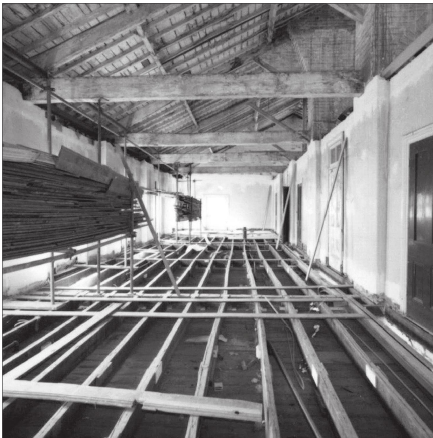
Figure 2.1: Cavity spaces between the joists below the floor on Level 3, looking east. Note the stack of floor boards on the scaffold at left (V. Pavlovic 1982).
