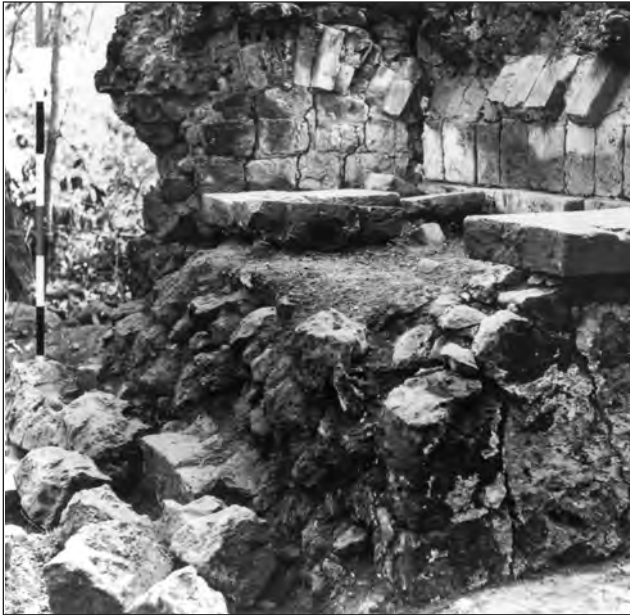
Figure 39. Collapsed western wall of the bakery showing solid fill construction beneath a barrel vault of masonry and brick.
