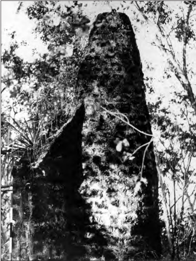
Figure 18. Married Quarters round chimney no.3 looking east. The positions of the vertical post, the principal rafter and horizontal beam on the external face are all discernible.
