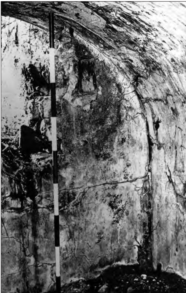
Figure 49. Interior of magazine.
