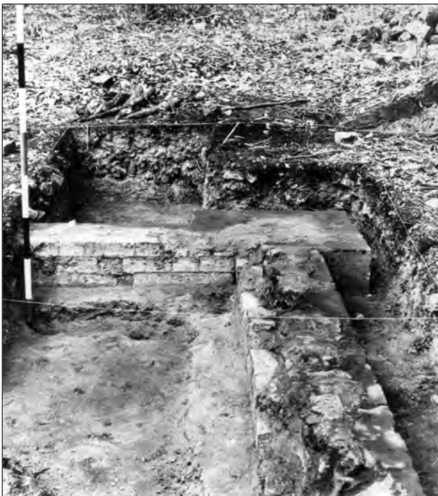
Figure 34. Excavation of VSD, western end, looking south. This shows how the stone and brick foundations have been set on wider concrete footings. Note how none of the walls remain above foundation level, indicating deliberate destruction of the building when the settlement was abandoned.
